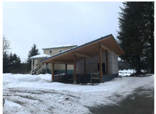
Exhibit 2-1: Cistern shelter during construction. Alternative water source provided by DRM for impacted property.
